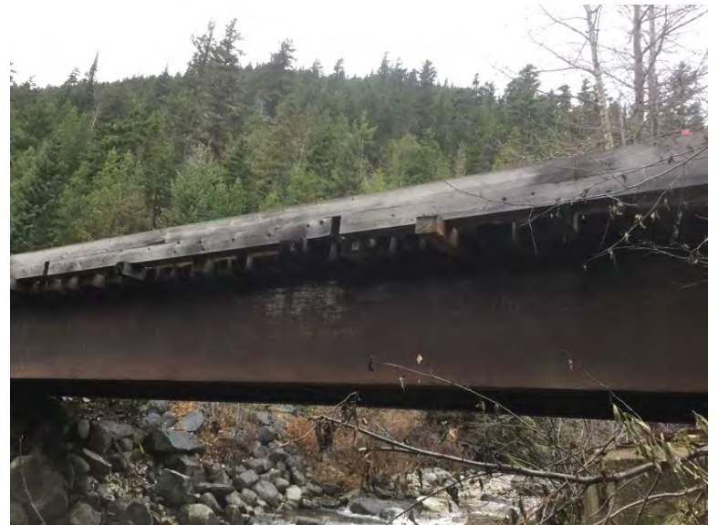
Guardrail and risers only fastened to a single in 6 locations along downstream end
