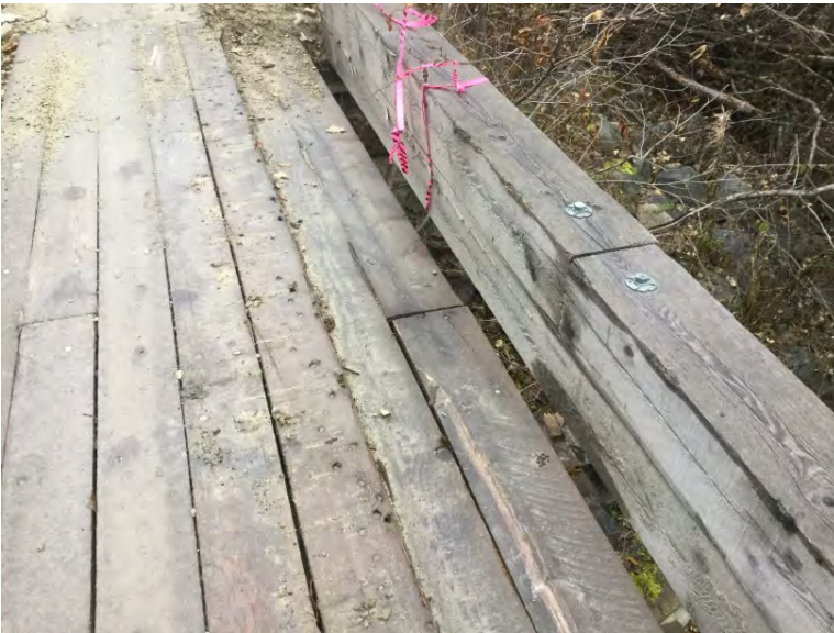
Downstream left bank missing appropriate length ties
