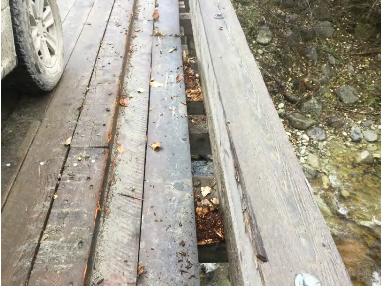
Tie condition downstream
