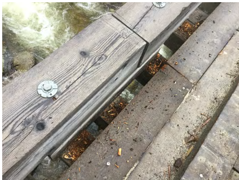
Tie condition upstream
