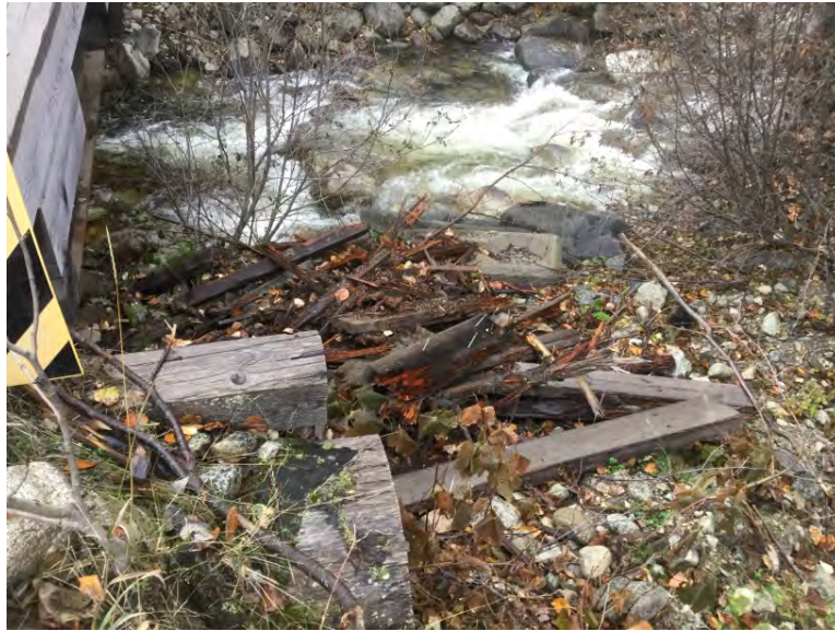
Old planks and subdeck spoiled at upstream left bank
