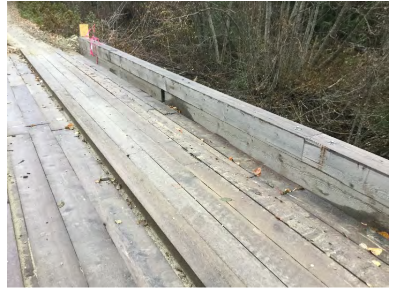
Downstream has full length risers
